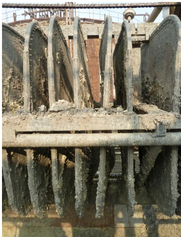
Figure 4. Corroded filter leaves.
