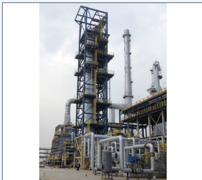
Fig: 1 IsoTherming® Reactor in Commercial Service
